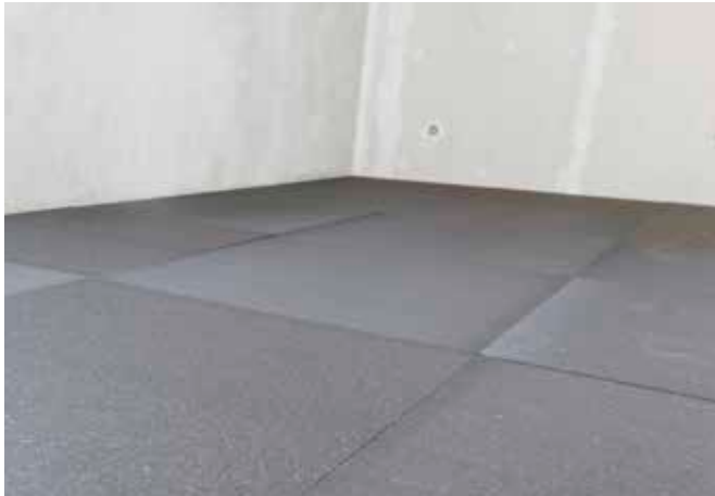
Full-surface laying of the bottom insulation, taking into account the existing supply lines.
