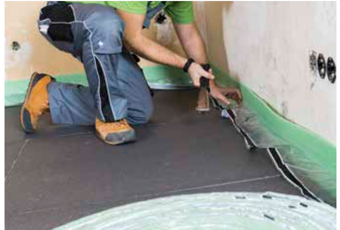
Fixing of the edge-insulation strips on all ascending parts. A reliable seal must be ensured.
